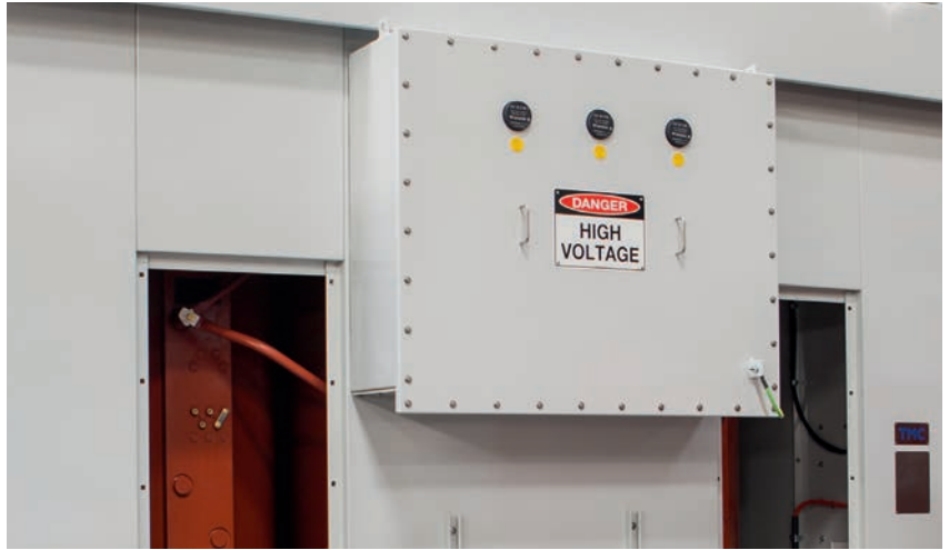
IP 43 (doors removed) showing Cable Box and front panel with infrared thermographic inspection windows
